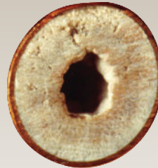
Pipe with scale build-up
